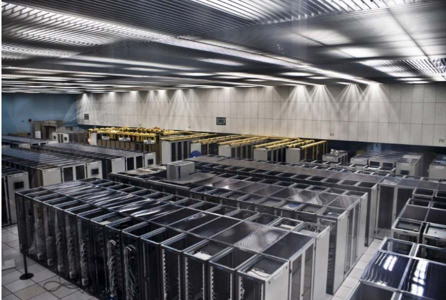
Figure 1.3 – A server room at CERN (Switzerland)
