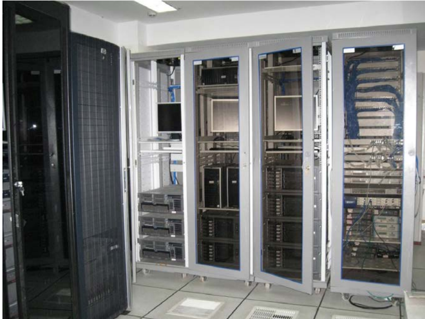
Figure 1.2 – Indian Railway 139 server room (self-hosting)
