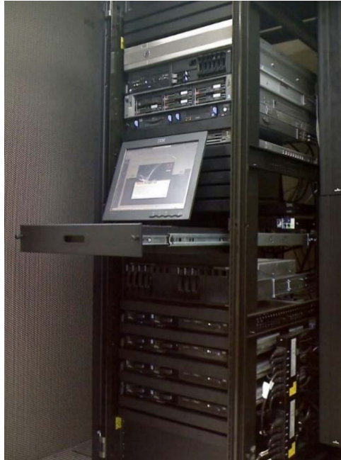
Figure 1.1 – A typical server rack, commonly seen in colocation
