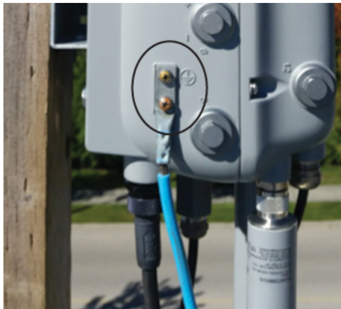
Figure 4-8 An Outdoor Access Point with Electrical Grounding (Photo Credit: Ian Procyk)
