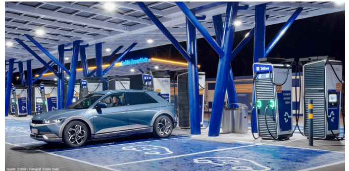
Fig. 1: Europe’s largest high-power charging hub with 26 CCS charging stations that allow a total of 52 vehicles to be charged concurrently [22].
